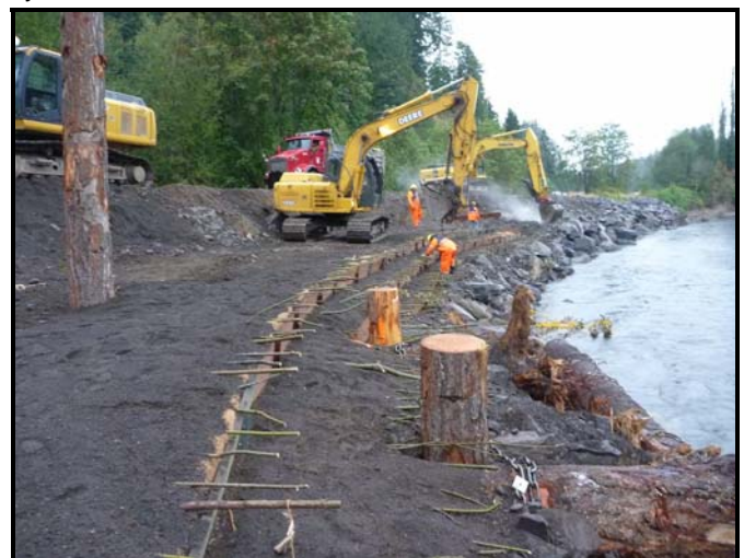
Cedar River bank stabilization, flood risk reduction project that uses boulders, large wood and rock ballasting to trap sediment, scour pools, create fish refuge, and establish riparian shade and cover. Photo Credit: King County.
